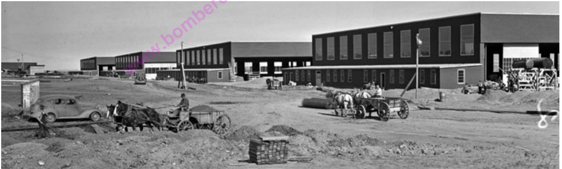
Horse-drawn wagons hauling loads of dirt during the construction of 2 Bombing and Gunnery School near Moose Jaw, Saskatchewan
