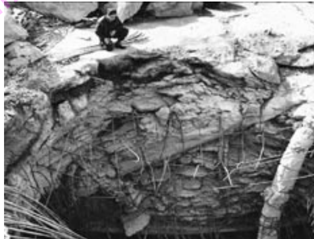
Grand Slam damage to the reinforced concrete roof of a submarine pen
